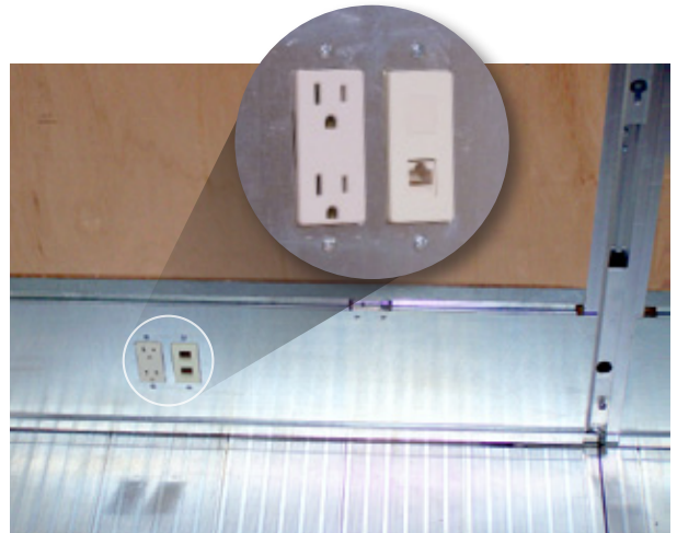
Electrical Access Panel - wired for both 110 volt and computer
